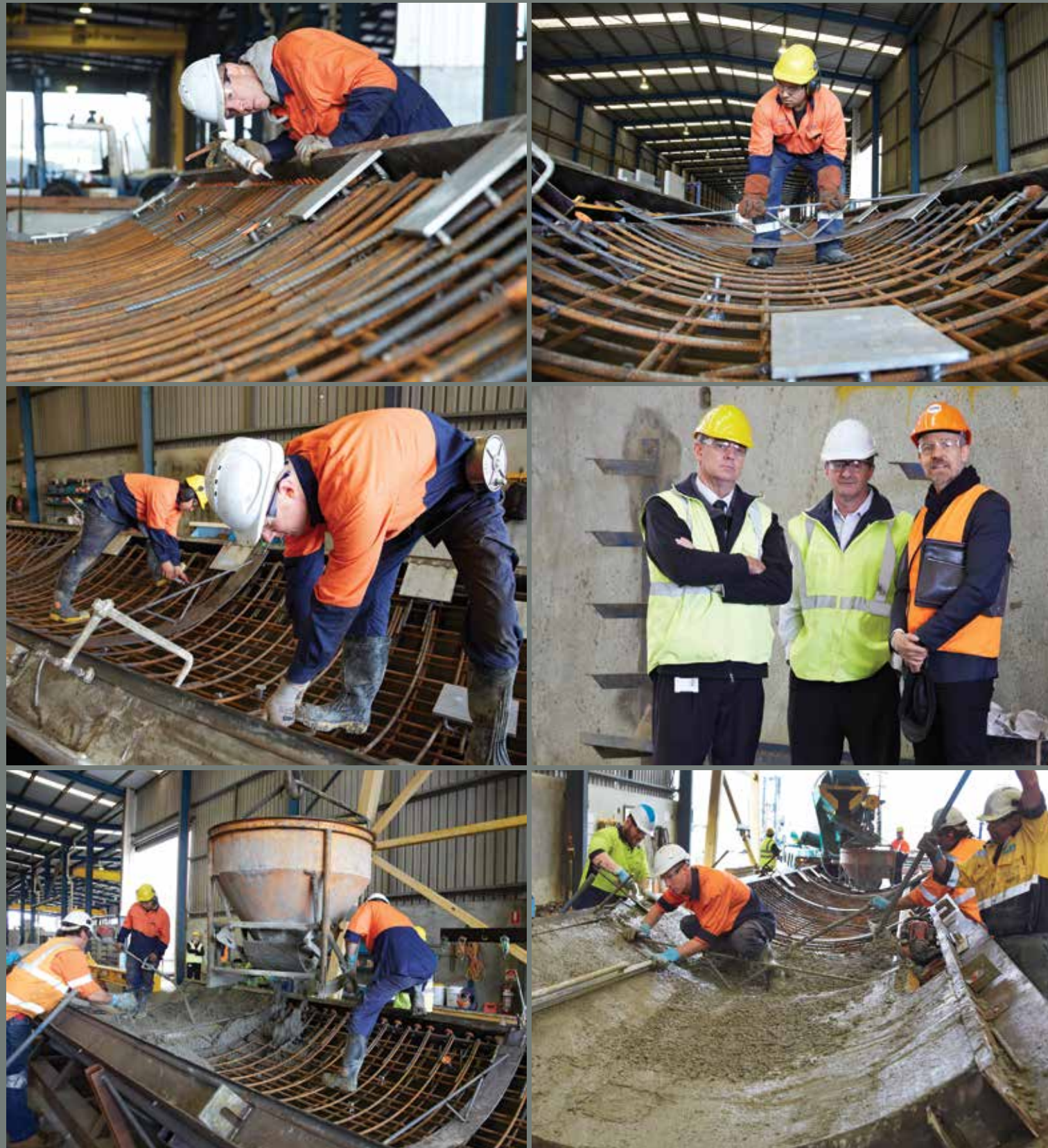
top row. Final inspection of the placement of the reinforcement in the steel formwork. Curved screeding guides are positioned at intervals.
