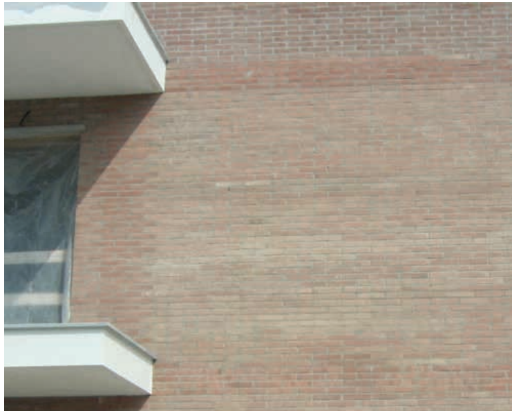
Darker banding across the slab sections due to cutting with dirty water.
