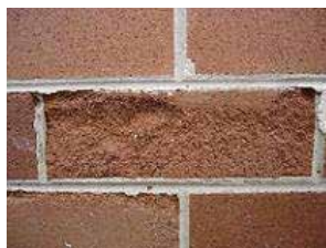
(a) dry press brick damage due to high pressure cleaning
