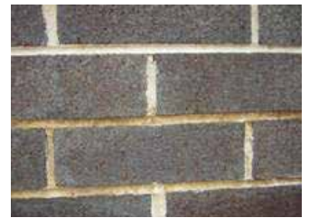
Iron Staining in Mortar Joints
